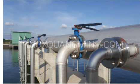
WASTE WATER TREATMENT SYSTEM / XỬ LÝ NƯỚC THẢI
